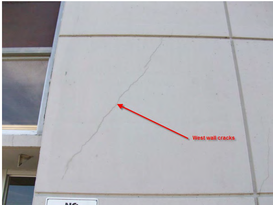
Photo 4: West wall cracks
